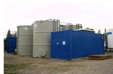
Biological groundwater treatment plant in Erkner (Berlin)
