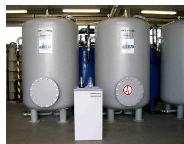
OXY-PURE® for catalytic wet oxidation at the site of a former coking plant in Zwickau (D)
